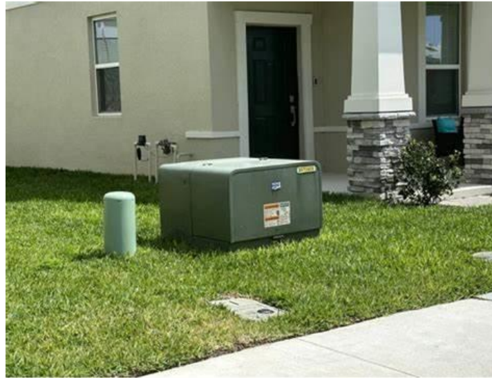
Figure 2 - Low Criticality Example: Residential Transformer
