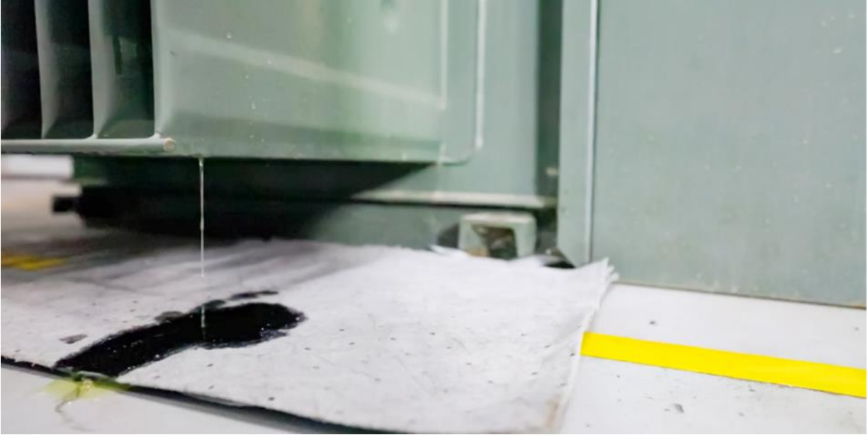
Figure 3 - High Health Example: Leaking Oil from Transformer
