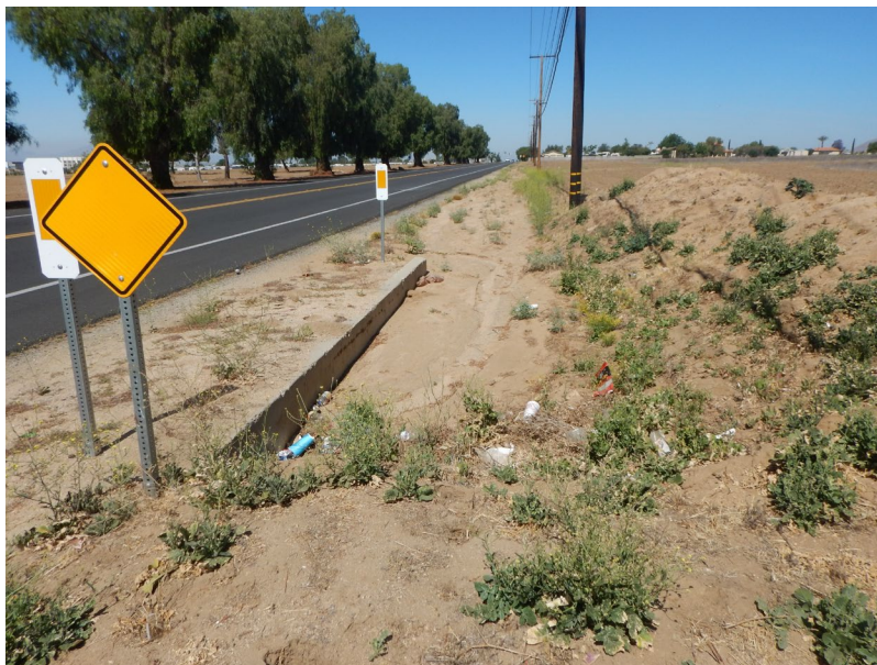
Photograph 3: View facing approximately west depicting the offsite concrete culvert which conveys flows from AF-1 south underneath Alessandro Boulevard, which is visible to the left.
