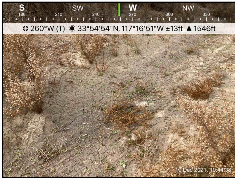
PHOTO 5: VP1 mud cracks near culvert. View is west (December 10, 2021).
