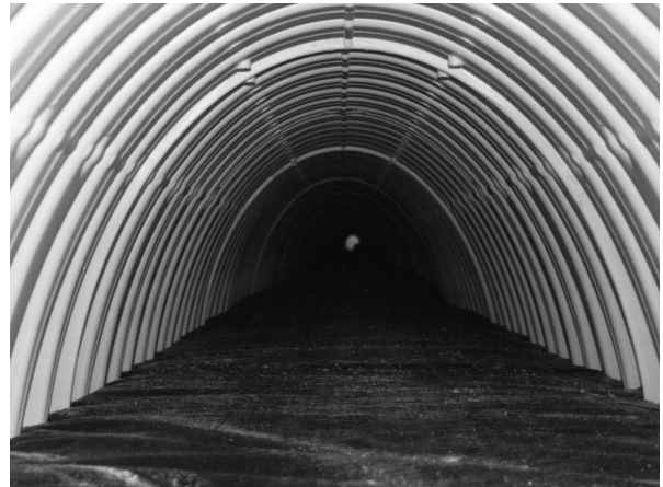
Looking down the Isolator Row
