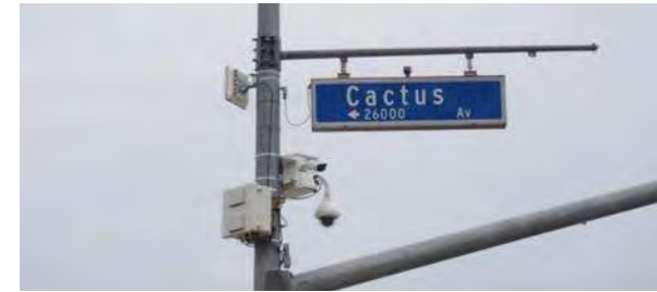
ITS allows the City to monitor different locations strategically and adjust traffic signals to improve flow.
